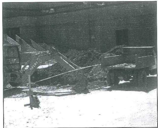
The construction area near the swimming and gym facilities. Renovation to the exterior of the building has continued with this project. Photo / Jerrick T. Adams
